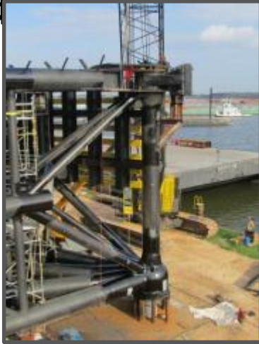
Sector Gate: Flood Control ~ 70,000 lbs
